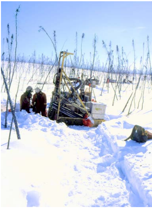
Figure 2.13: Winter exploration in Eagle Plains: setting up a portable drilling rig. (Photo: Yukon government)
