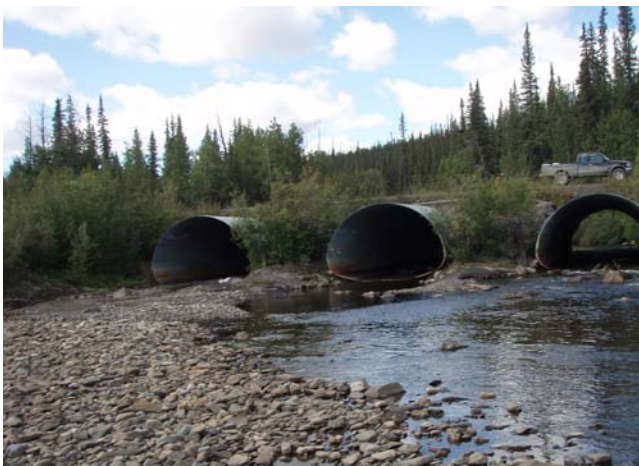
Figure 2.26: Culverts at the Davies Creek crossing of the Dempster Highway. (Photo: A. von Finster, DFO)
